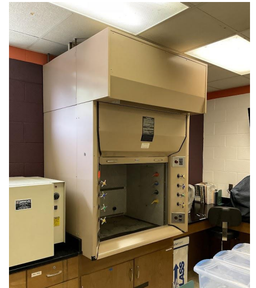
AREC Fume Hood to be replaced
